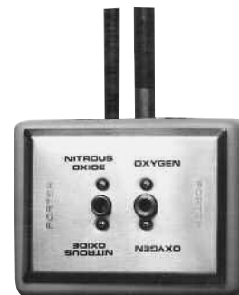
6200-1 WITH 6250K N 2 O/O 2 OUTLET STATION (EXPOSED)
